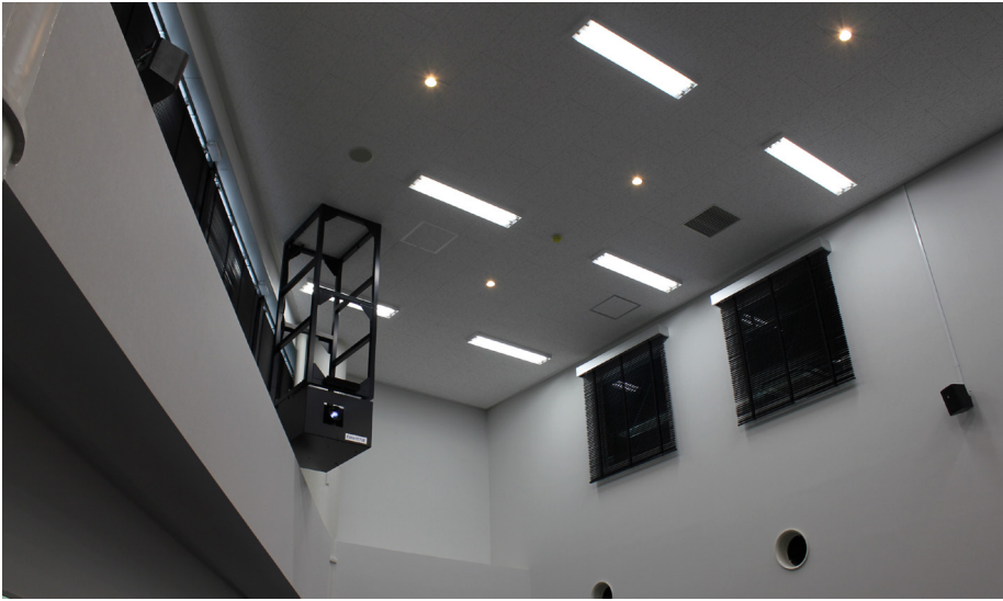
▲ The Christie HD10K-M projector installed at Yamagata University's conference room.
