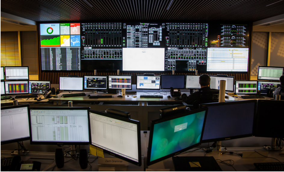
▲ Invenergy recently upgraded its control center with a Christie solution comprising a tiled LCD panel video wall and a Christie Phoenix content management system.
