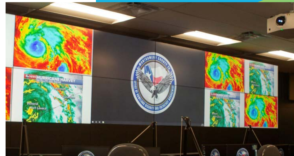
^ Montgomery County's EOC relies on a 12-channel video wall of Christie Extreme Series LCD panels in a 2 x 6 array, with content delivery by Christie Terra SDVoE solution via 10G Ethernet.
