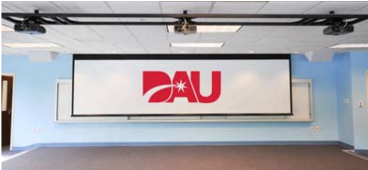
A growing trend on campus are the DAU TriZenter classrooms that use 3 ceiling mounted DS+305s, projecting onto a 20' screen.
