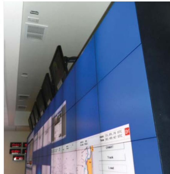
▲ Custom design and engineering helps with ventilation.
