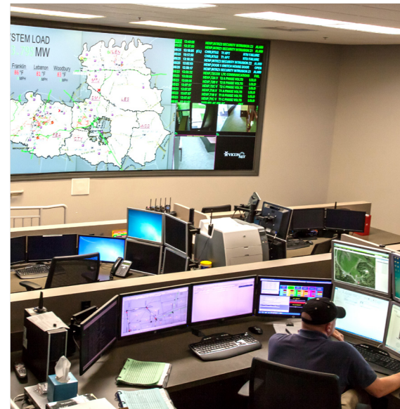
▲ A view of the control room, with the focal point of the room being the updated, dynamic video wall.
