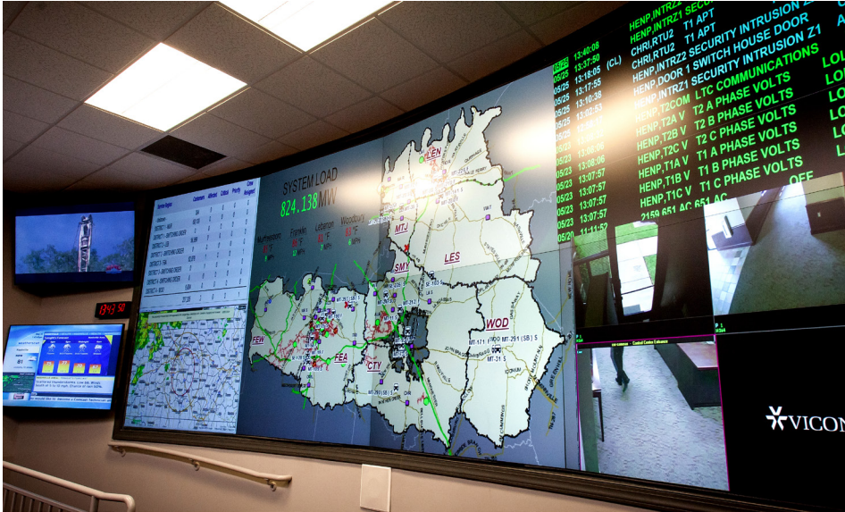
▲ MTEMCC's control room video wall.
