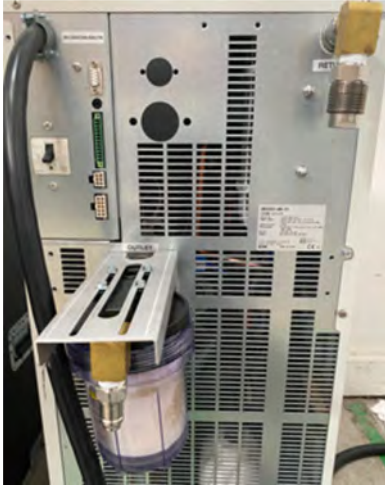
Rear of chiller
