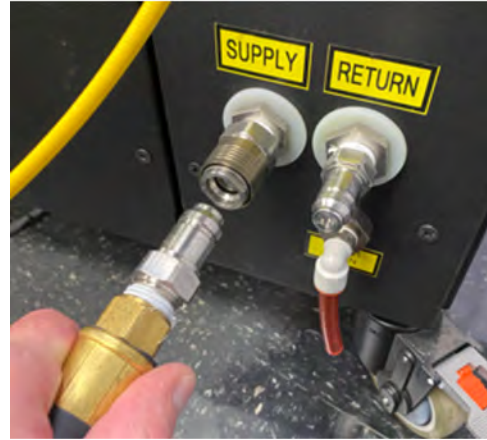
Rear of laser rack
